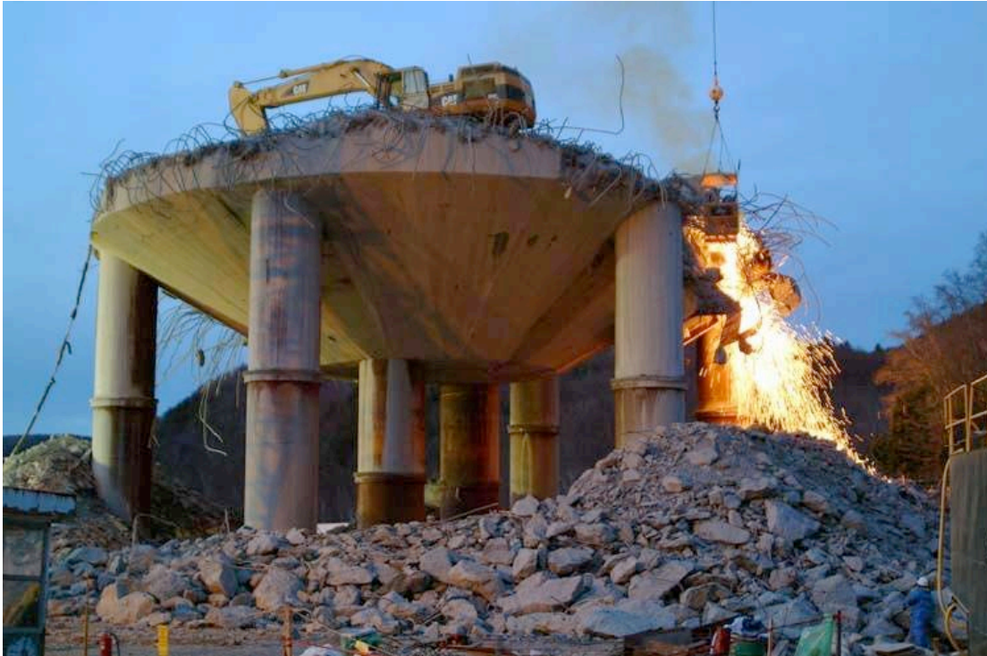
Lancing (Cutting) Rebar in the Lower Section of the Reactor Support Structure
