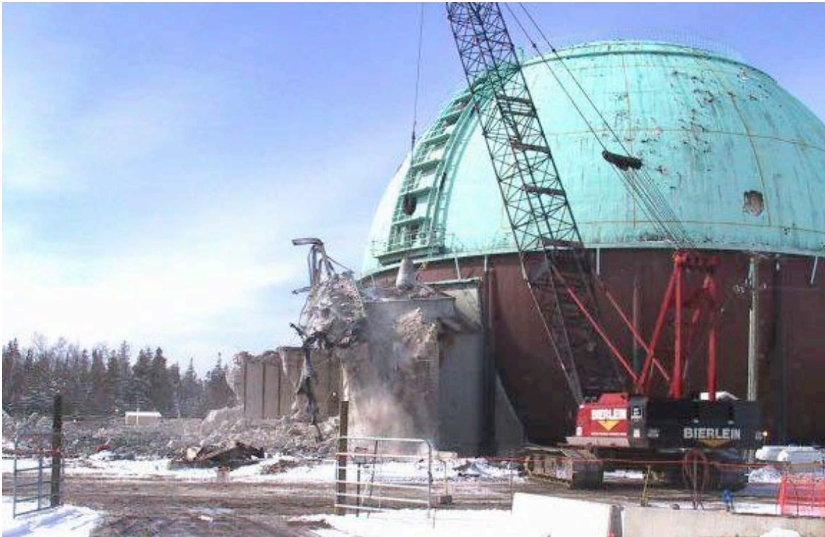
Final Wall of Former Control Room being demolished with 17,000 Pound Wrecking Ball
