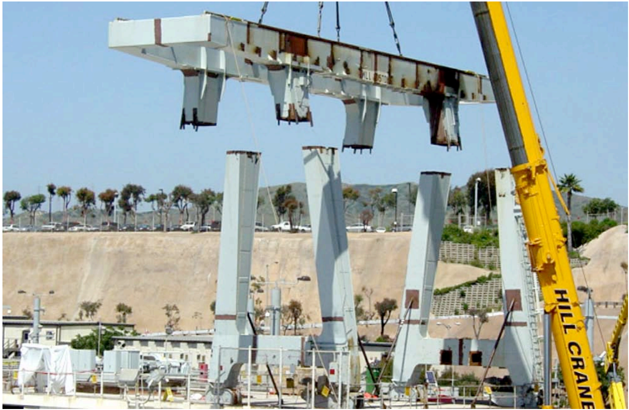
SONGS Unit 1 Gantry Crane - The top girder is slowly and carefully lifted off and lowered to the ground after being cut free.
