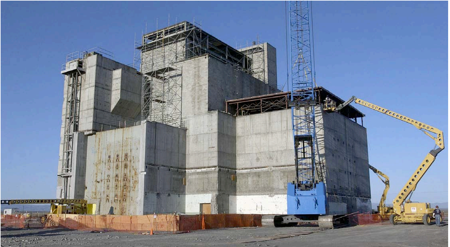
Construction of a New Roof on the Hanford H Reactor for Interim Safe Storage
