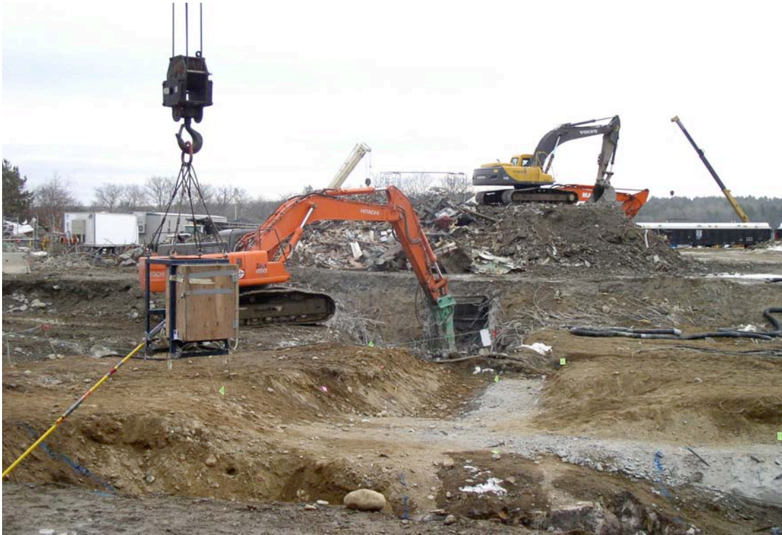
Remediation and Final Survey Work in Former Spent Fuel Pool Building Area
