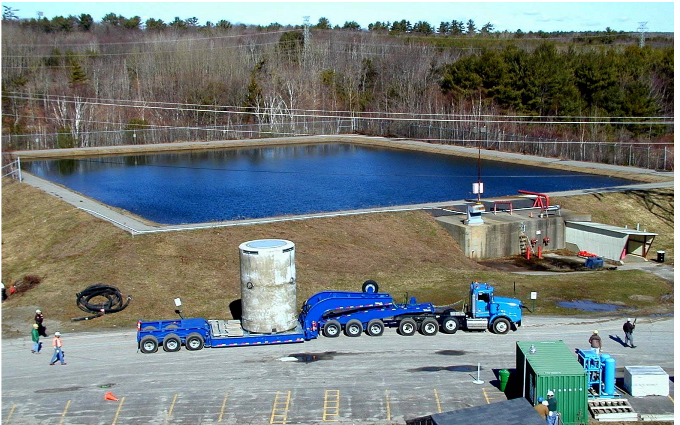
Transfer of 4 th and Final Vertical Concrete Canister of GTCC Waste to the ISFSI
