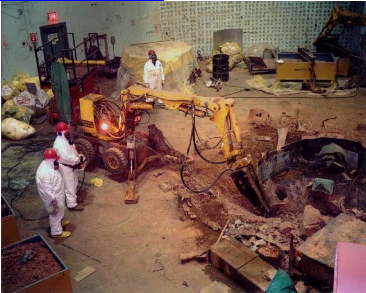
The BROKK excavator being used to break up the concrete base of the biological shield structure in containment at the CP-5 facility.
