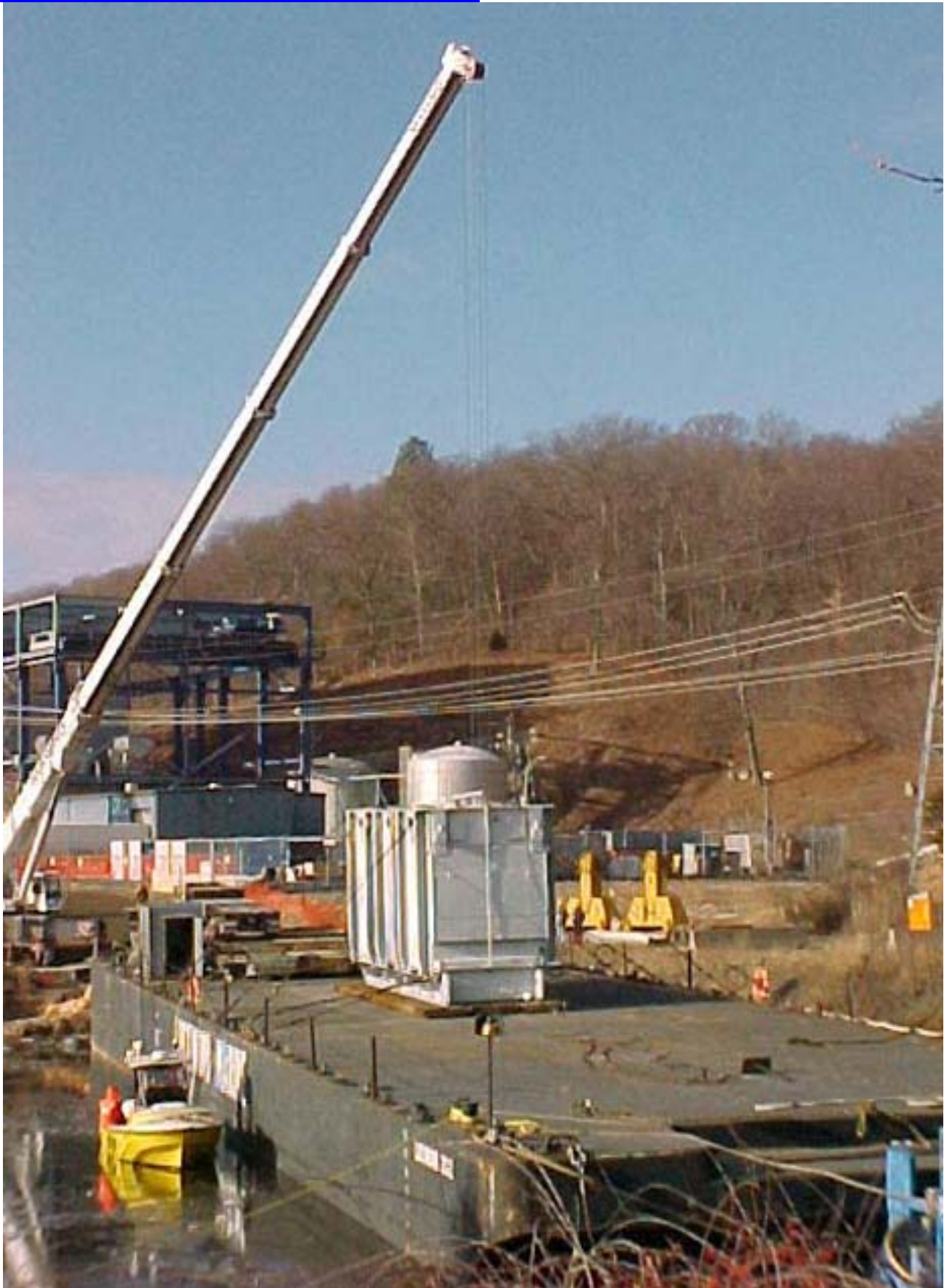
Transformer Barge Shipment
