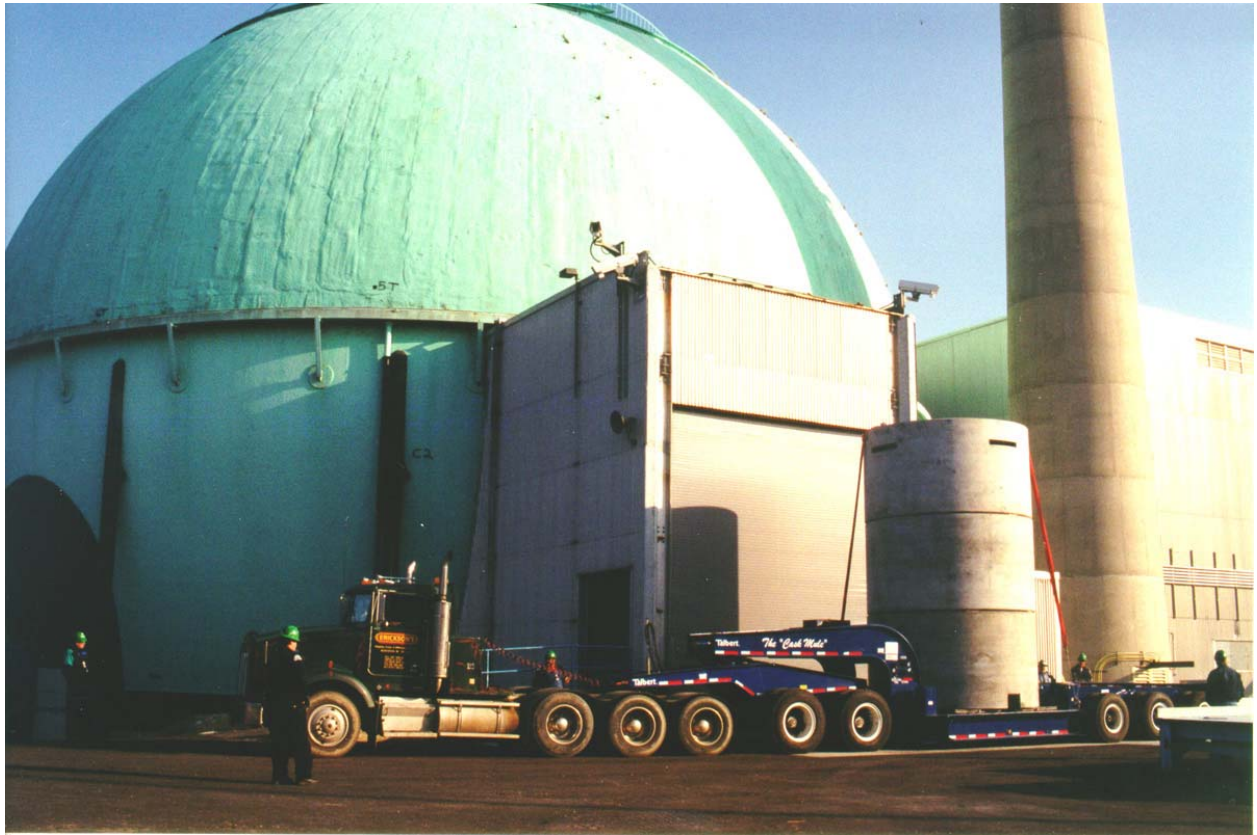
A heavy hauler is used to move a concrete overpack from the containment sphere to the dry fuel storage pad
