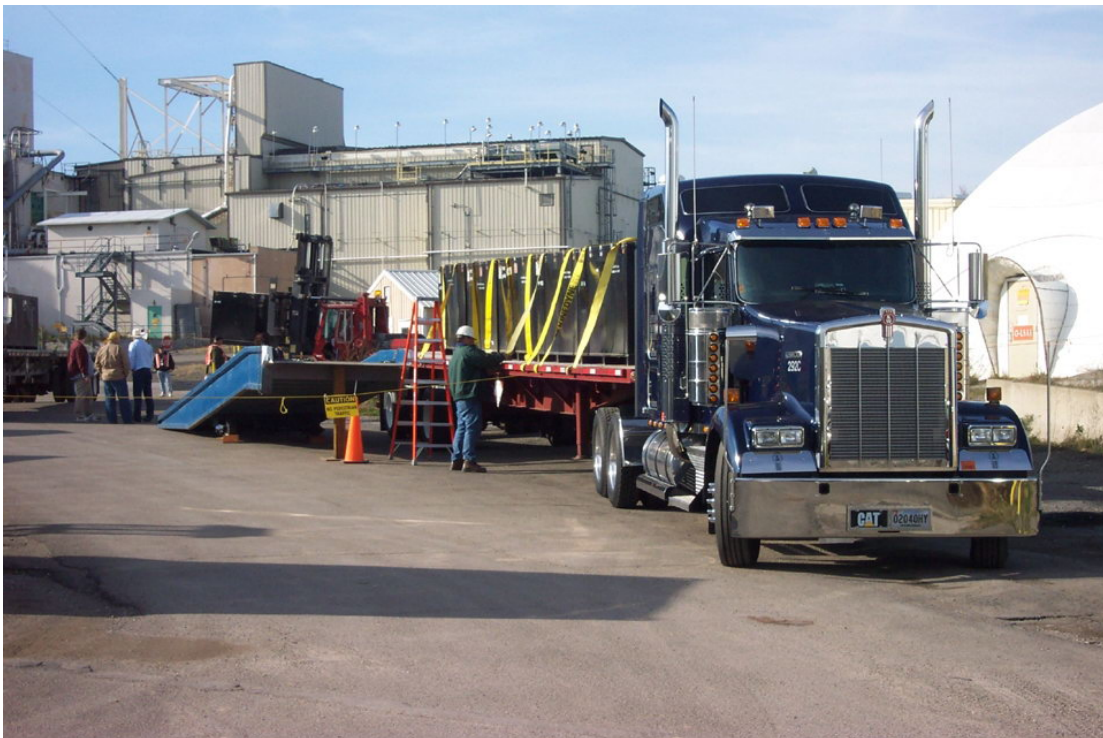
Large scale debris is being size-reduced and packaged with a remotely-operated Brokk TM
