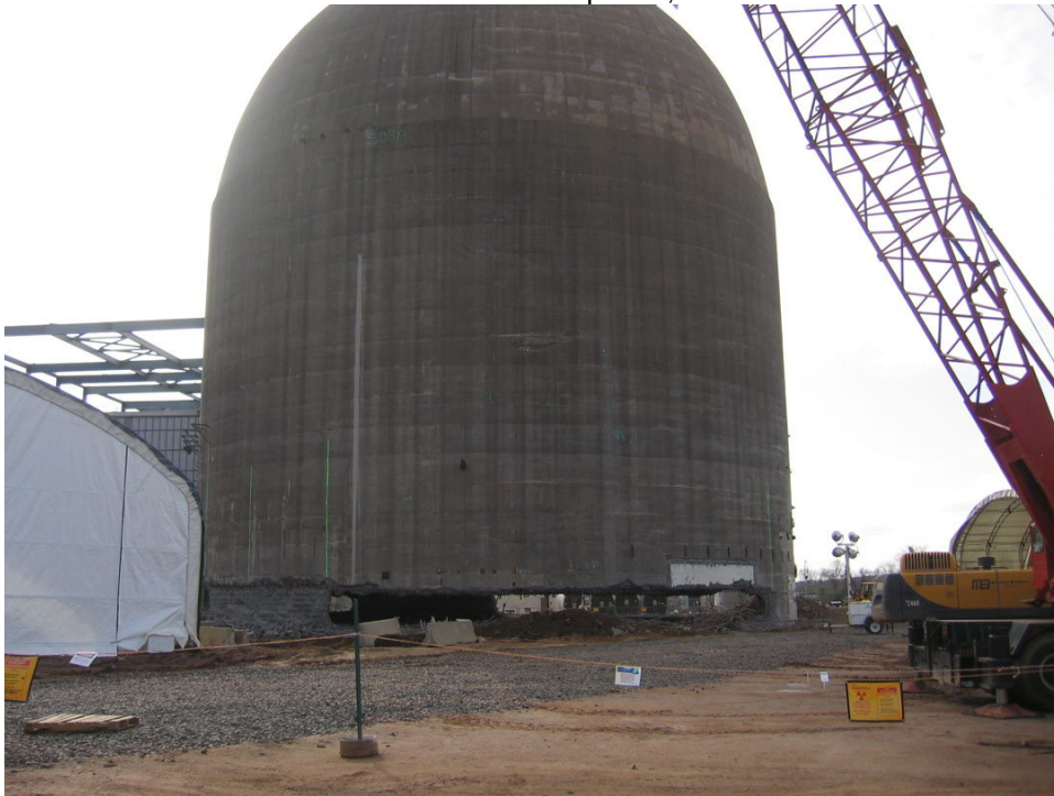
Containment with the first round of cuts on the bottom of the structure
