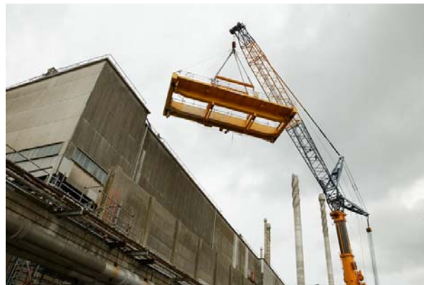
Redundant crane section after removal through the roof of the Magnox Swarf Storage Silos
