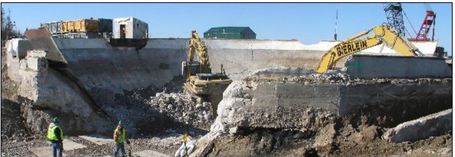
A road was built to allow equipment to travel down into the containment sphere and remove debris.
