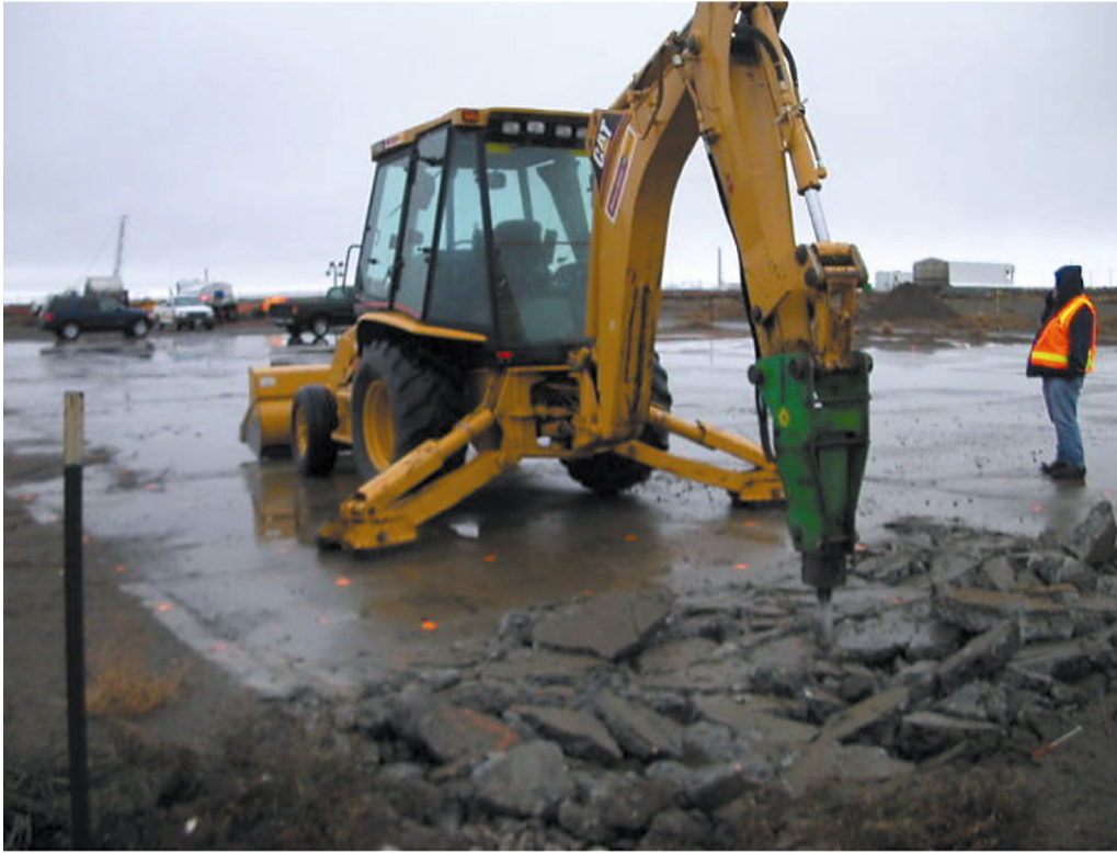
A “concrete cracker” breaks up a large slab so that crews can excavate a buried waste pipe, a precursor to some of the first cleanup work on waste sites in Hanford’s central plateau area.
