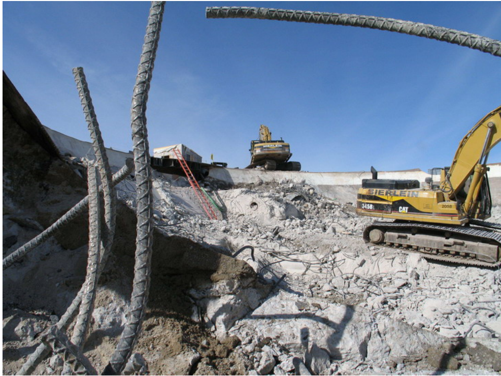
After using explosives to soften the concrete and rebar inside the containment sphere, workers mined and packaged the debris for disposal.
