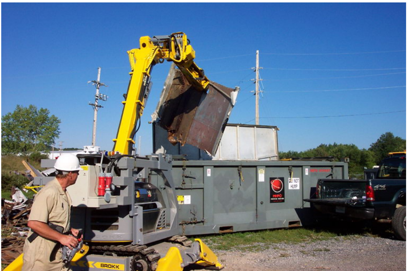
Waste boxes loaded with LLW are being secured on a truck for off-site disposal
