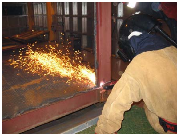
Plasma cutting of redundant ISO containers at the new Metals Recycling Facility
