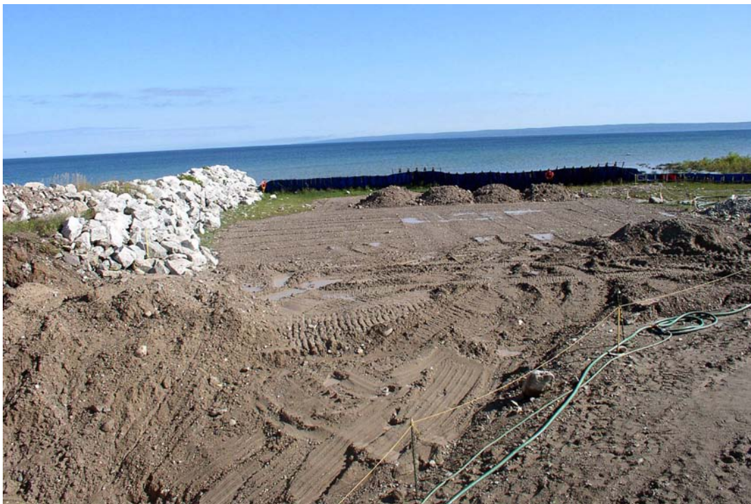
Remediated canal returned to its original contour - much like it was before Big Rock Point was constructed
