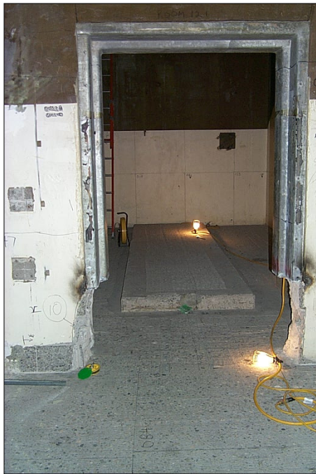
Safety Injection Pump Room
