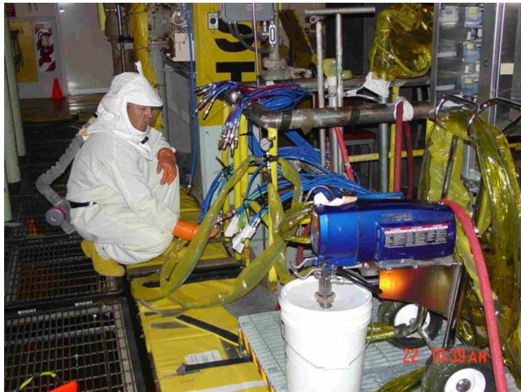
A pipe fitter adjusts hoses that fed a specially formulated cement mixture into the discharge chute between the K East Reactor and the K East Basin at Hanford.
