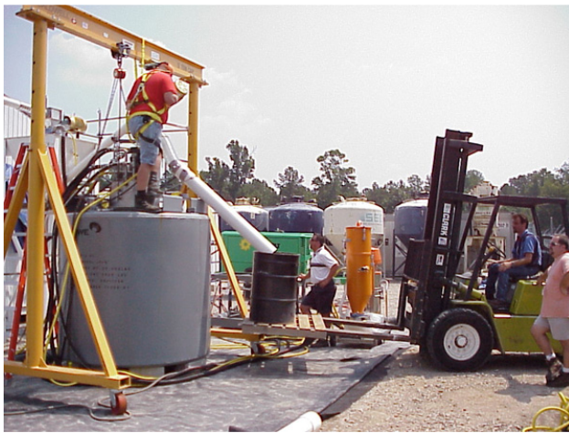
Mock-up of the SBW solidification system at the vendor's shop.
