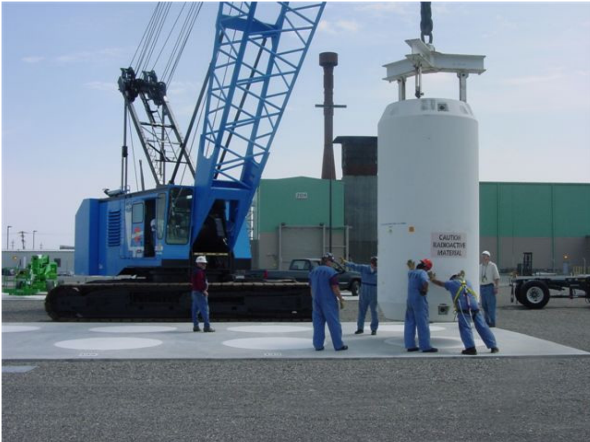
Spent nuclear fuel from the Fast Flux Test Facility is placed in an Interim Storage Area at Hanford.
