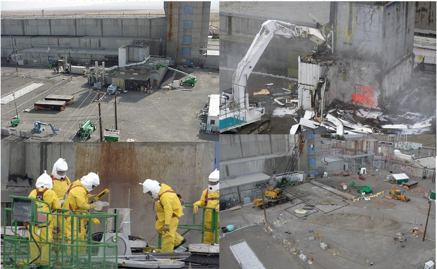
Photos of the 233-S Plutonium Concentration Facility; before demolition (upper left), during concrete shearing operations (upper right), during concrete cutting operations (lower left), and after site stabilization (right).
