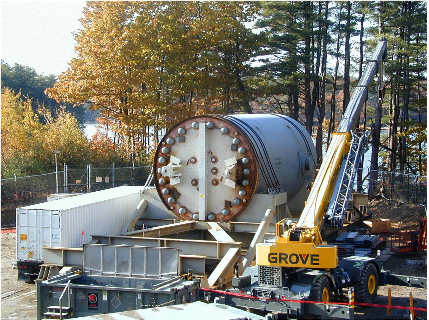
Maine-Yankee Reactor Pressure Vessel in Storage Container Outside Containment
