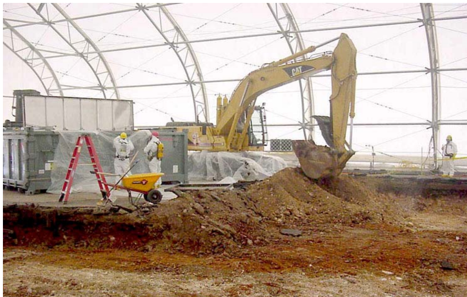
Although most of the contaminants are limited to the first 2 feet of soil at the 903 Pad, up to 4 feet of contaminated soil is being removed for packaging and disposal as low-level mixed waste.
