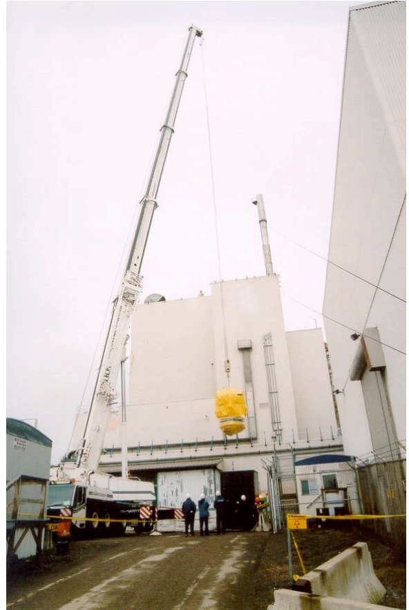
A 200-ton mobile crane is used to move this Extraction Cell-2 tank into a waste box.
