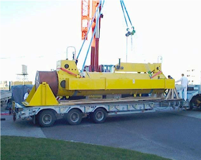
AT1 (FBR former reprocessing facility) Removal after using in the decommissioning of high activity cells of the ATENA carrier.
