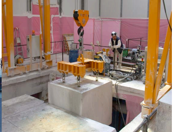
EL4 HWGCR in Brittany, decommissioning under progress, evacuation of concrete blocks (6 to 8 tons) from the irradiated cells examination building using diamond cable wiring.
