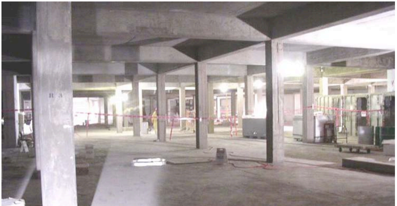
Once home to thousands of liters of plutonium liquids, gloveboxes, tanks, and processing systems, B771 decontamination is nearly complete and demolition is scheduled for this summer.
