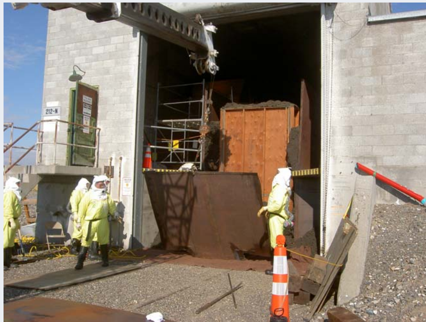
Figure 2 - Workers uncover and remove a large crate containing transuranic waste at a degrading World War II structure, as part of facility cleanout, November 2006.
