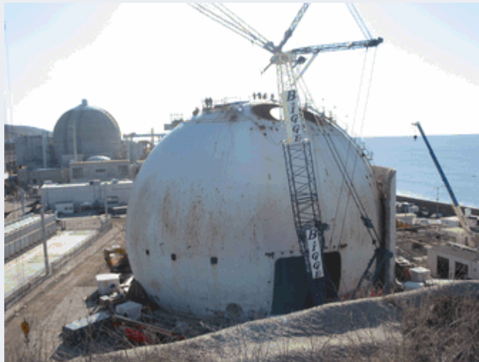
(1) San Onofre Nuclear Generating Station (SONGS) Unit 1 Containment Sphere prior to the dismantling of the one-inch thick 140-ft diameter steel plate structure.
