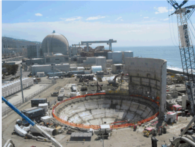
(2) San Onofre Nuclear Generating Station (SONGS) Unit 1 Containment Sphere foundation after sphere removal
