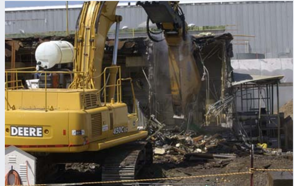
Demolition of the highly contaminated 232-Z Plutonium Incinerator Facility at the Hanford Site was a highlight of D&D activities completed this past summer.
