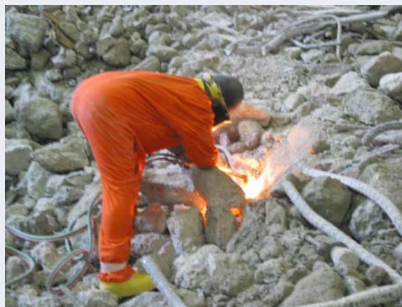
Crushed concrete area and torch cutting of rebar at SONGS to resize material to fit into intermodal and/or lift-liner containers.
