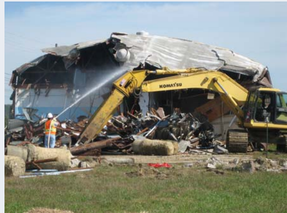
The 11,000 square foot X-105 Electronic Maintenance Building was recently demolished in October 2006. The building was constructed in 1957 and had been vacant since 2001.
