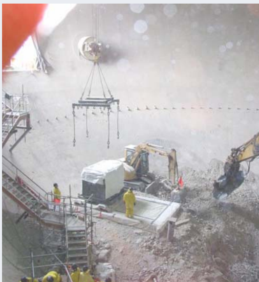
Excavators inside SONGS reactor building containment hammering concrete rubble near the bottom of the steel liner as this work is nearing completion.
