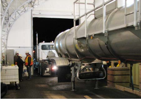
Fluor Hanford workers ready a tanker truck to remove a load of the contaminated water being drained from the K East Basin, February 2008.
